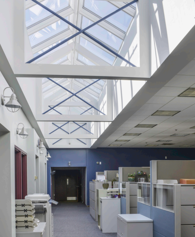
Two VMS Ridgelights replaced two failing translucent panel systems to transform the US Ironworks Facility in Ohio.
