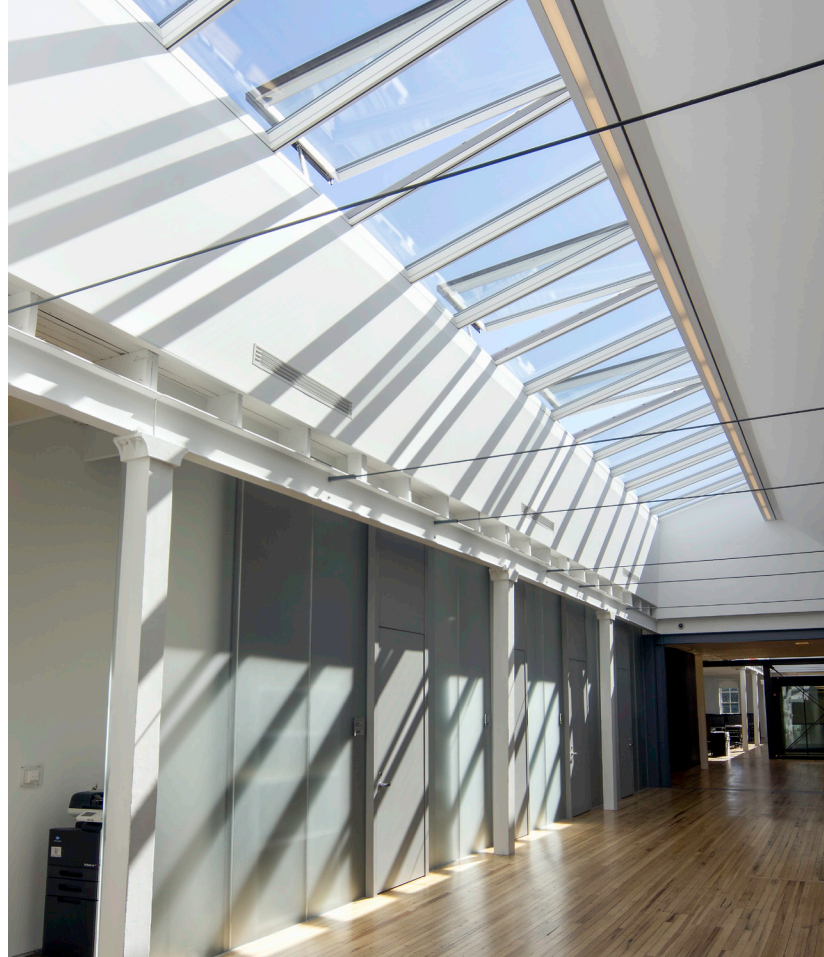
VELUX Modular Skylights were chosen to modernize the repurposed third floor space of Cornell University's College of Architecture.
